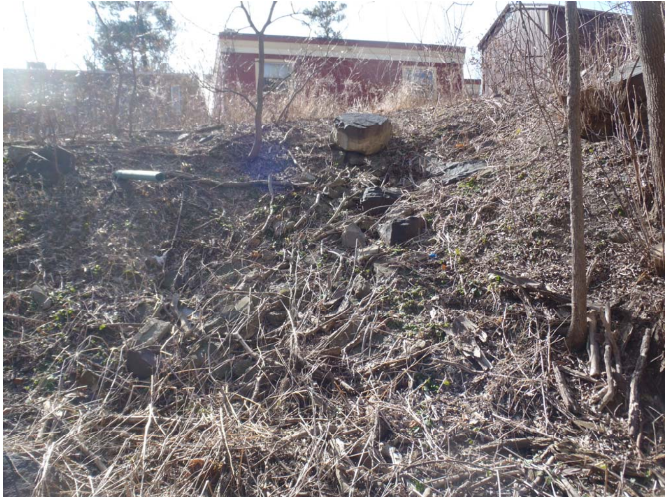
Photo 1: Presumed Location of Natural Drainage Swale and Unknown Subsurface Drainage Outlet
